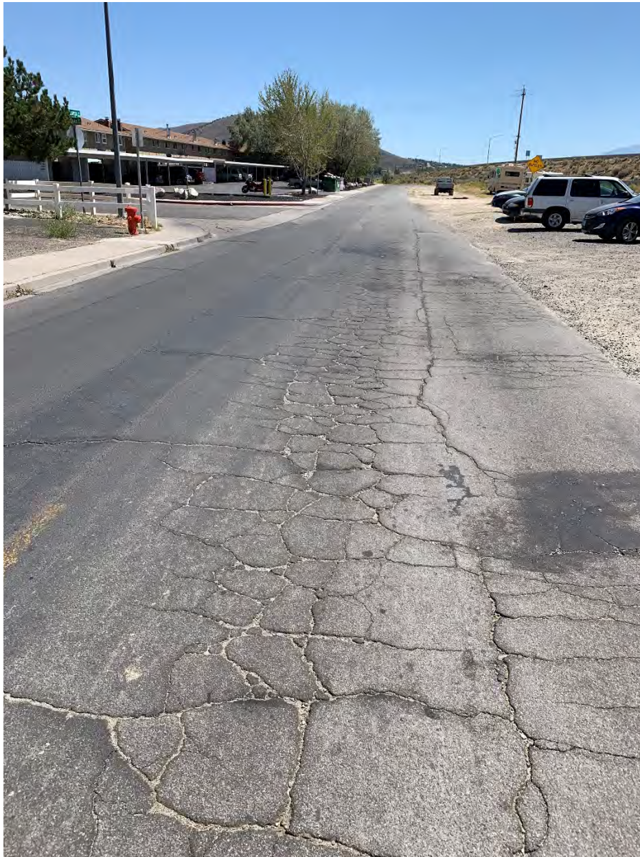
Figure 6. Pavement in Very Poor condition category (PCI 40-26).
