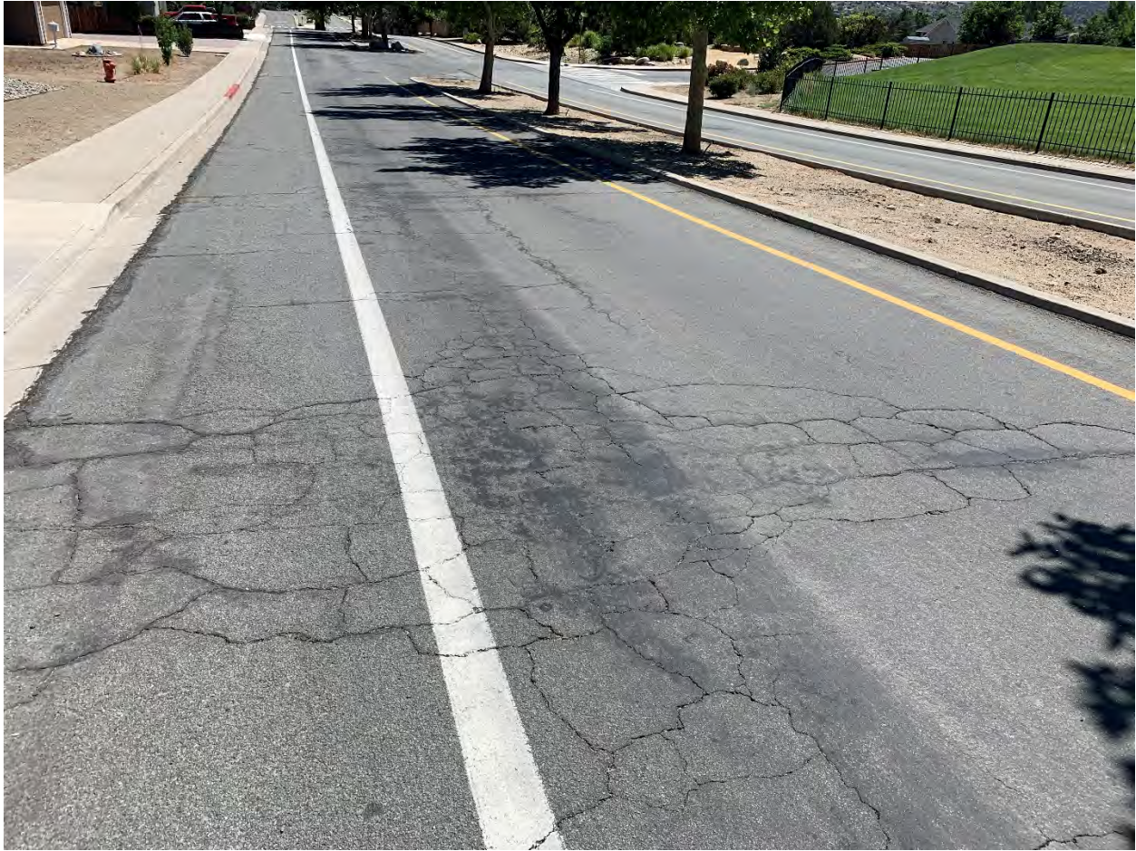
Figure 5. Pavement in Poor condition category (PCI 55-41).
