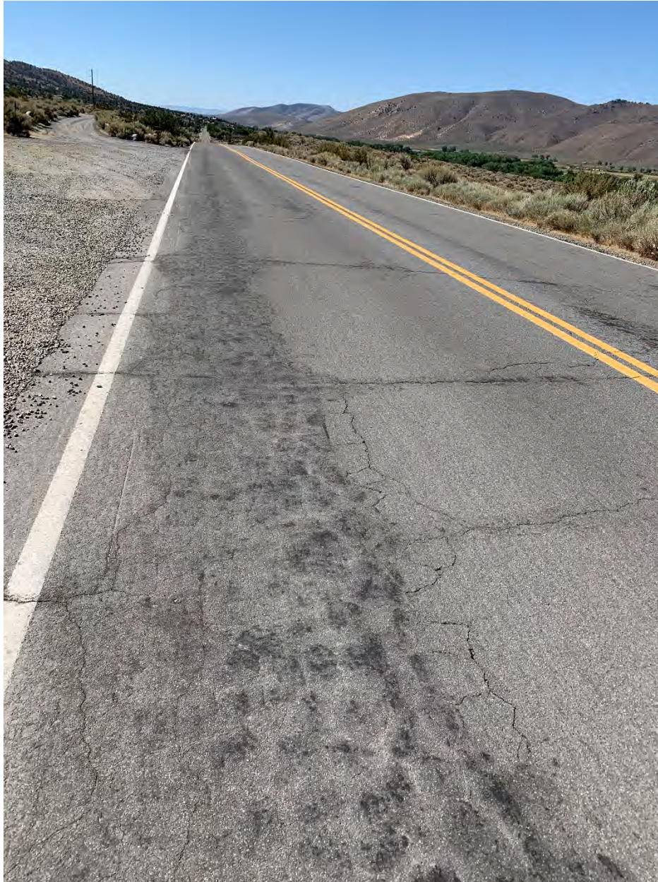
Figure 7. Pavement in Serious condition category (PCI 25-11).
