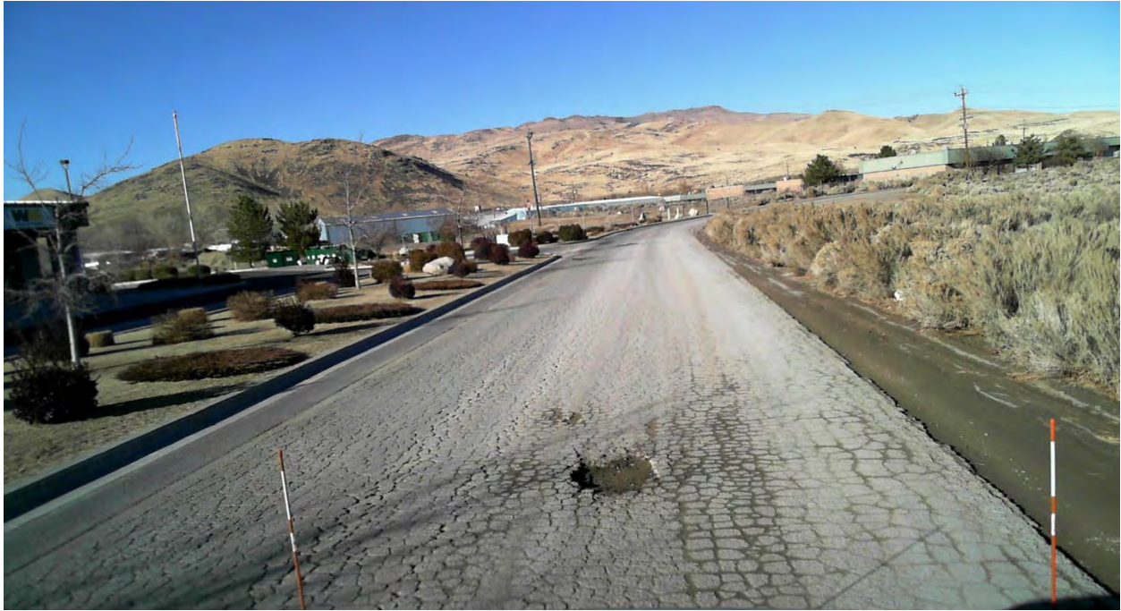
Figure 8. Pavement in Failed condition category (PCI 10-0).
